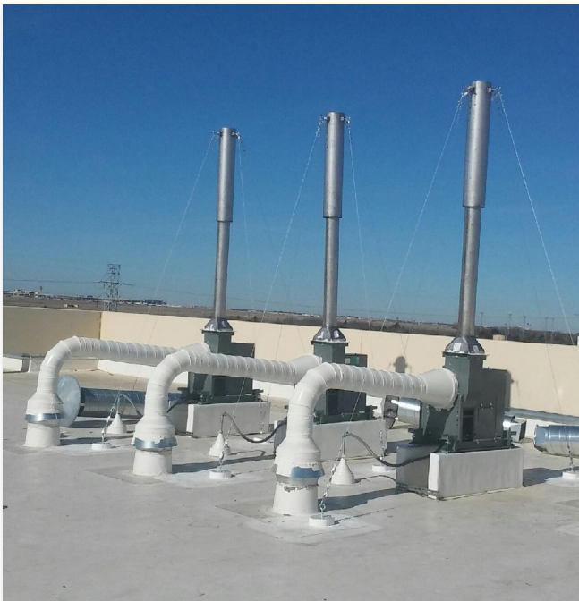
Typical Class II BSC Exhaust System
