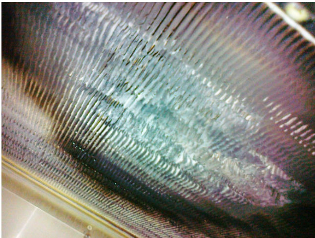
Charred HEPA filter
